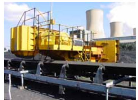
Stockpile Reclaim Feeder on site
