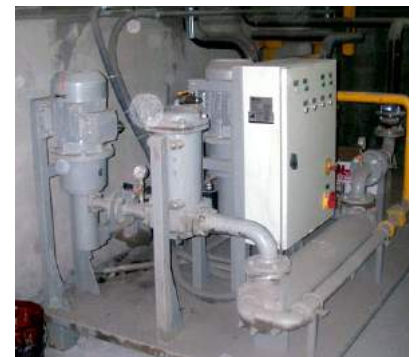
Retrofitted lubrication Symetro Gear system with local control panel.
