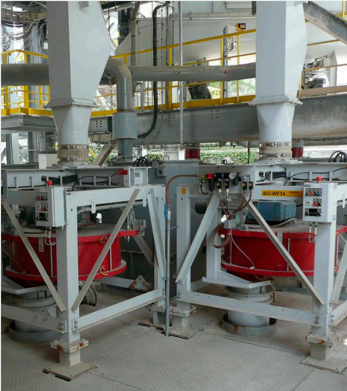
Blending installation at the finish mill of a cement plant in Germany.
