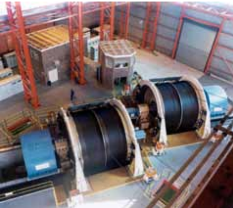
Ø 5.7 m Electrically Coupled BMR Hoist - Moab Khotsong
