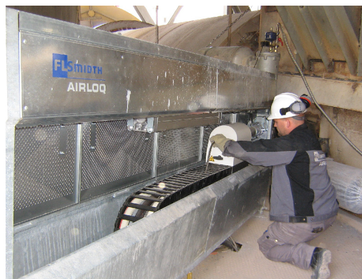
Fig. 4 After the expiration of the system warranty period, the customer will take over the responsibility for servicing the gas analysis system.
