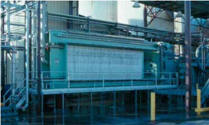
Overhead Beam Filter
