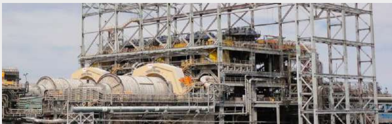
Ball Mill, Pumps and Manifolds
