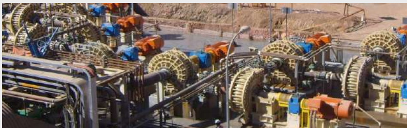
High Pressure Pump Train
