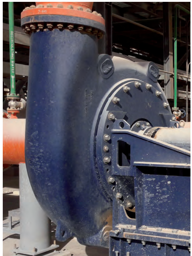
millMAX pump installed at a phosphate plant in Saudi Arabia
