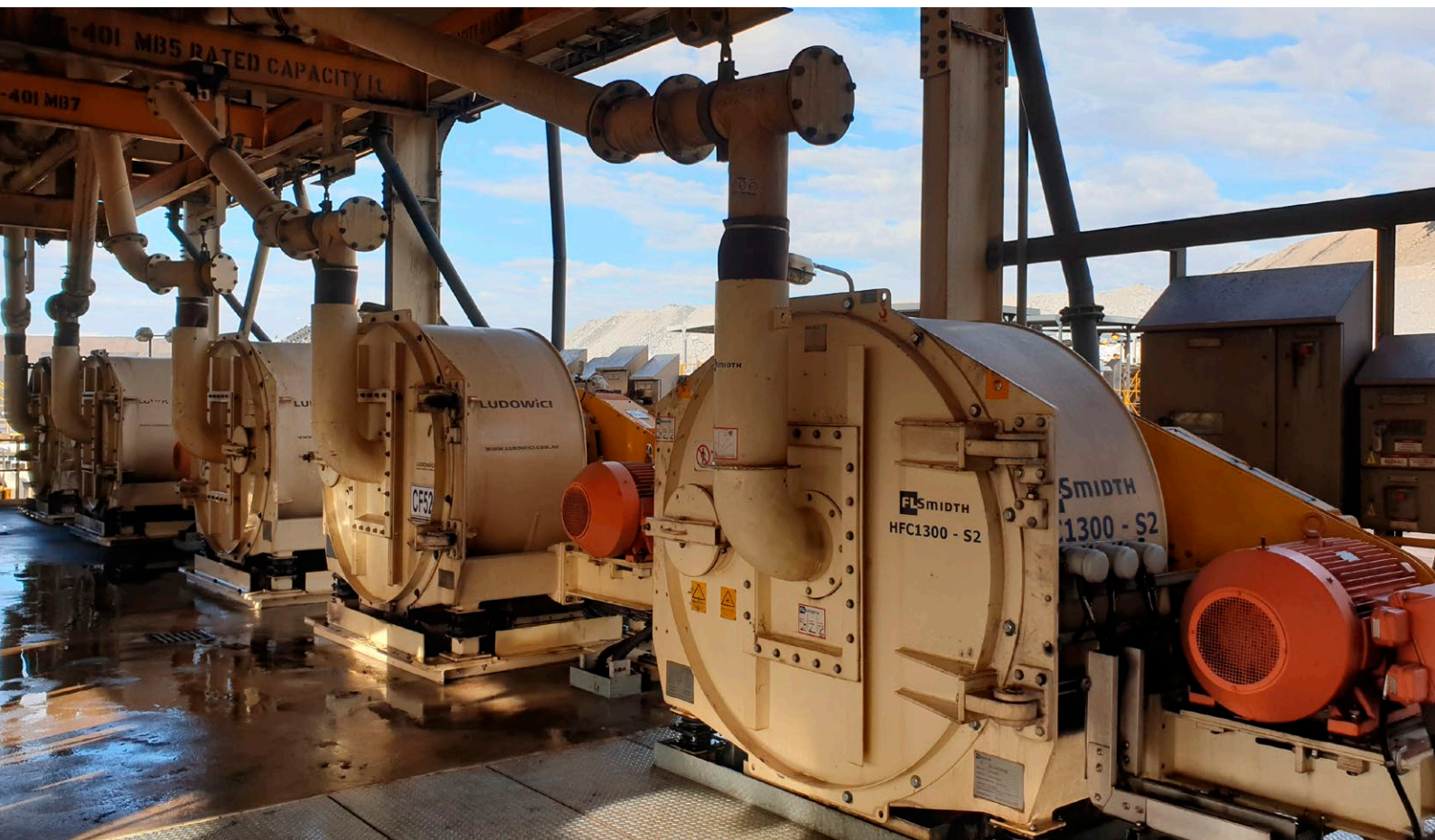
Above: Whitehaven Coal's Maules Creek Mine, in the new South Wales Gunnedah basin, was chosen as a trial site and the HFC1300 Series 2 Fine Coal Centrifuge was installed in the plant circuit in parallel with four existing Series 1 units.
